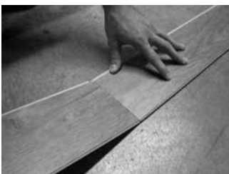
Fig. 3 – Angle end tongue into end groove on planks in the initial row.
