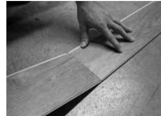
Fig. 3 - Angle end tongue into end groove on planks in the initial row
